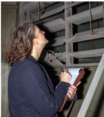
Heating, ventilating and air-conditioning inspections during existing building commissioning often include documenting the condition and functionality of fans and louvers.
